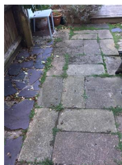
Stone slabs Weathered
