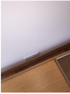
White plastic, double socket Good condition
