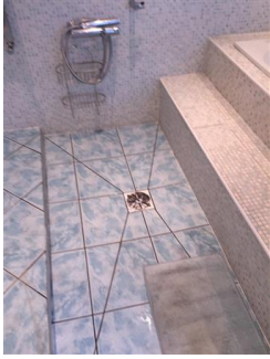
Wet area in the front of bath area
