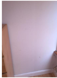
Scuffs and scratch to lhs wall
