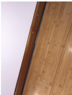
Gap between skirting and floor
