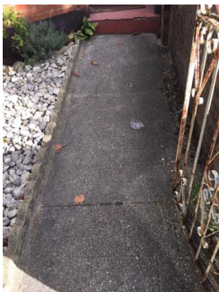
Concrete path Weathered
