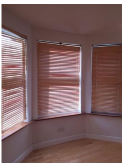
Wooden Venetian blind with pull cord Good condition Lhs bay blind is not working
