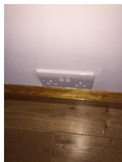
White plastic, double socket Good condition
