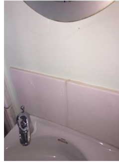
White tiles above basin
