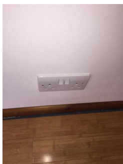
White plastic, double socket Good condition
