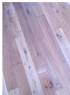
Line scratch near centre of the room
