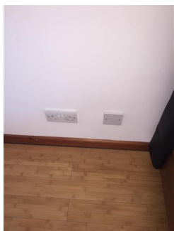
White plastic, double socket Good condition
