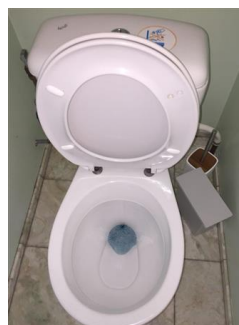
Internal view Clean
