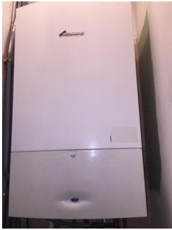
Worcester white boiler Good condition
