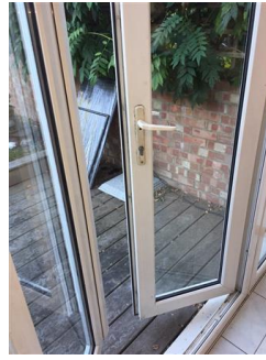
White UPVC frame, double glazed double patio door, white lever handle with cylinder lock, leading to rear garden Good and working condition
