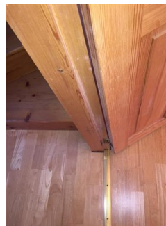
Brass threshold Good condition
