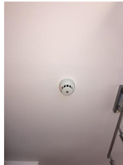
White plastic heat and smoke detector Good and working order
