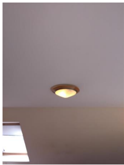
Frosted glass dome Good and working order
