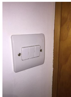
White plastic triple light switch Good condition
