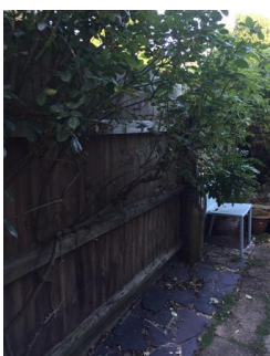
Concrete uneven slabs to the side
