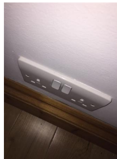
White plastic, double socket Good condition
