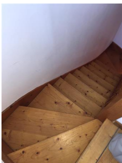
Wooden stairs Tarnished, moderate usage
