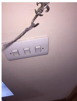
White plastic triple light switch Good condition
