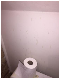
Yellow splash stains above cistern
