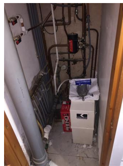
Internal view Needs cleaning inside
