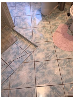
Blue / white, square tiles Cracked tiles near entrance
