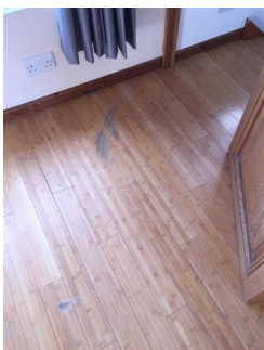
Light wood floor boards Scratches in many places
