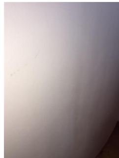
Light scuffs to staircase
