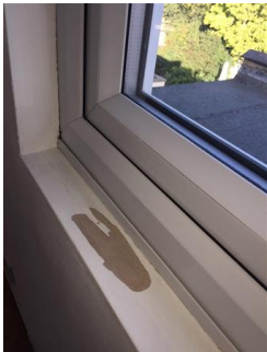
White painted window sill Chipped
