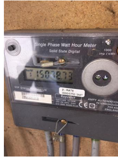
Electric meter located outside the house Reading: 15078.73 (rate 1) S/N: Z05E005310
