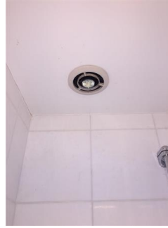
1x spotlight above shower area Not working
