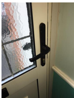
White UPVC frame Cracked to joinery
