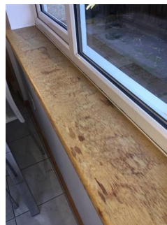
Wooden window sill Ring marks, discolourations
