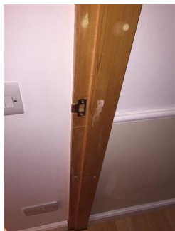
Light wood stained door frame Few chips and scratches in places Visible repairs
