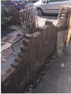
Brick wall to rhs of the house Aged
