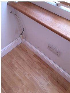
Loose cable to lhs
