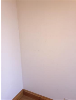
Settlement crack to corner
