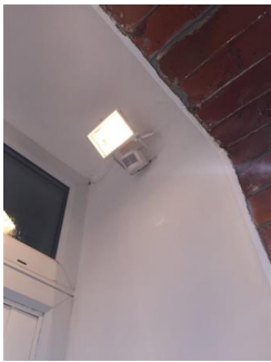
Halogen light, white framed Working
