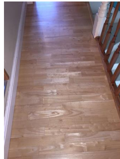
Light wood floor boards Long scratch to first floor
