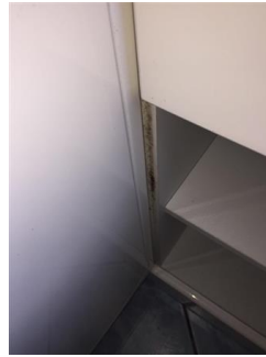
Needs light cleaning to the edge
