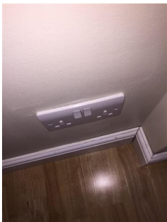
White plastic, double socket Good condition
