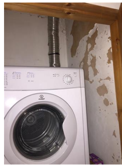
Heavily peeling paint to white painted walls
