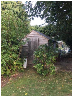
Wooden shed to lhs of the garden Weathered Padlock attached, key handed over to tenant
