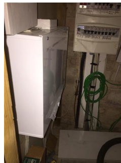
Internal view Fuses box and alarm box
