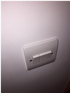
White plastic triple light switch Good condition
