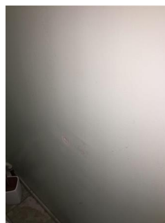
White painted walls Visible repairs to rhs wall
