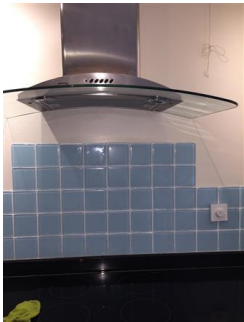
Blue, square tiles to lhs of the kitchen, above hob and sink area Good condition
